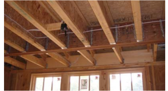
Highlighting many "green building" principles, this home includes energy-efficient windows, material-efficient joists and composite structural beams.
