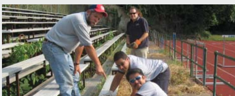
BOWA's DC/Arlington/Alexandria and Customer Service Teams cleaned, landscaped and performed minor repairs at the Duke Ellington Field in Washington, DC.
