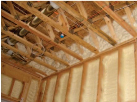
A layer of air-sealing spray foam applied within the walls and at potential leak points in the attic helps to minimize air leaks in the building's shell - a critical first step.
